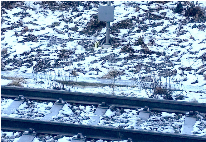
XT-3HD reader mounted track side, The Swedish Transport Administration, Sweden.
